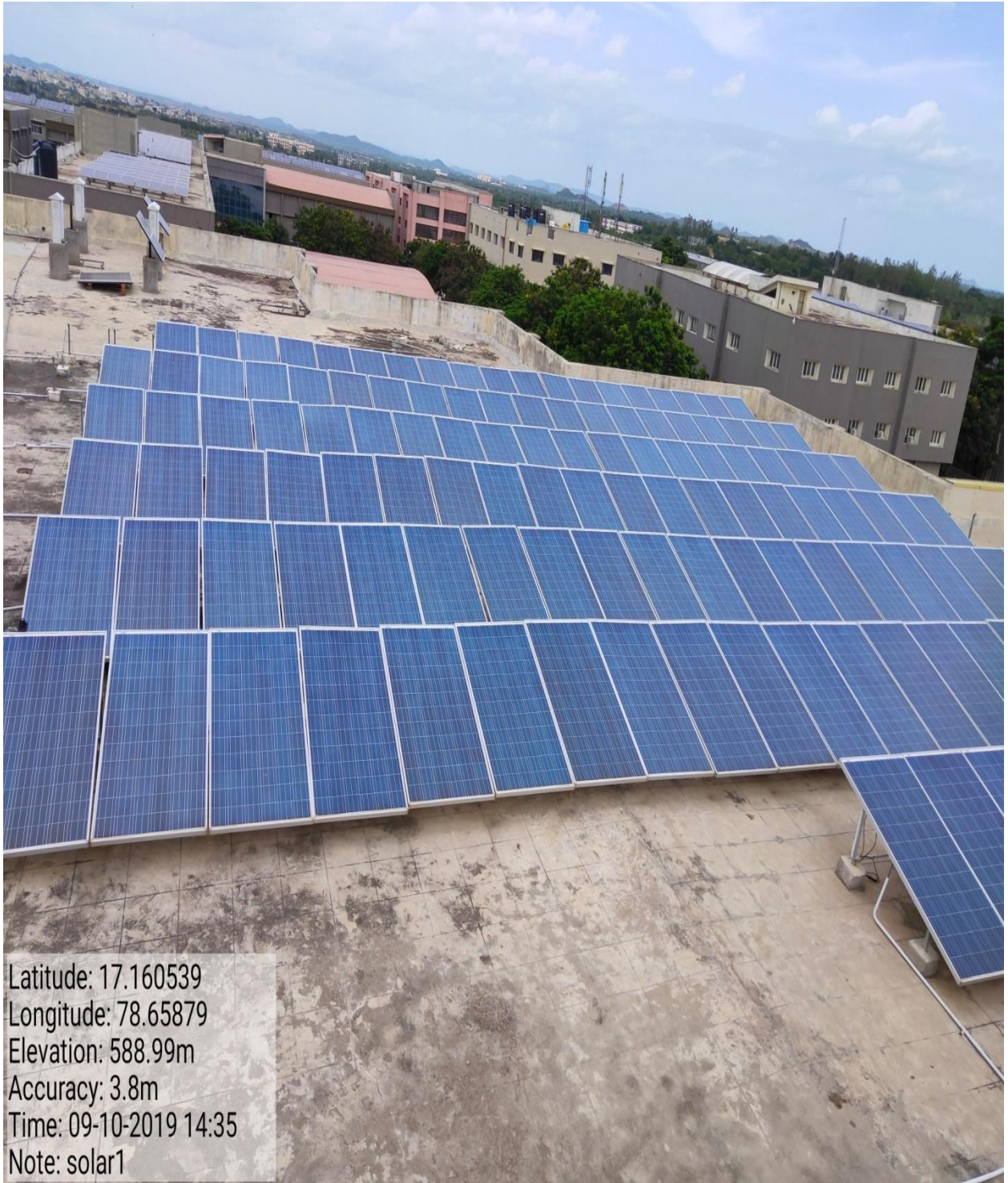
Solar plant which is situated in GNIT Campus
