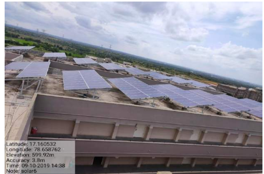
Top View of The Solar Plant On Block B& C Building
