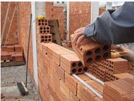
Clay blocks (sometimes called clay block brick) being laid with an adhesive rather than mortar
