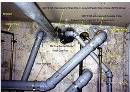
Plastic pipes penetrating a concrete floor in a Canadian highrise apartment building
